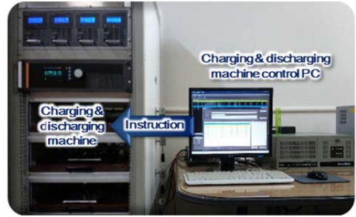
(b) Charging and discharging machine.
