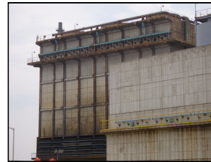
(c) Hot water pump of steel plant
