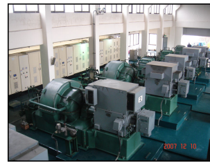
(a) Blower of sewage disposal plant
