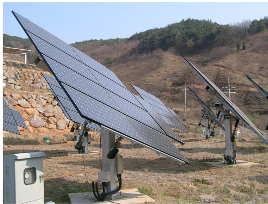
(a) PV tracking system.
