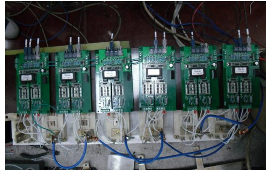
Fig. 14. The inverter for experimental test bench.
